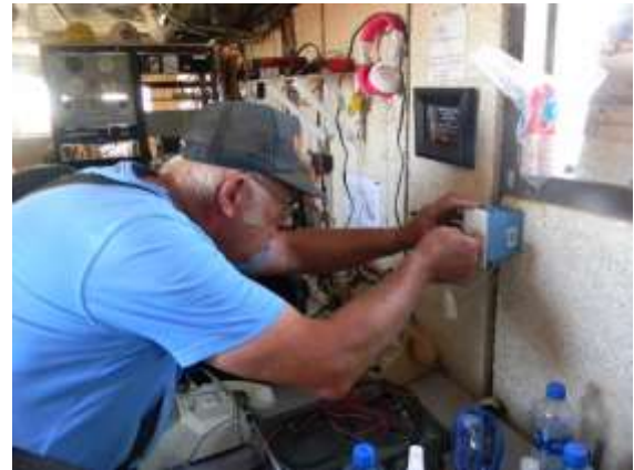
Figure 12 Ed Corn installing the hard phone line outlets in the comm. trailer
