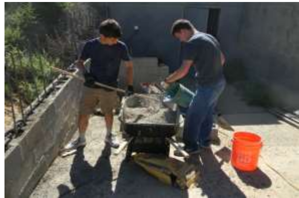
Figure 9 Hans Gaensbauer and Alex Schor mixing concrete for the bunker ramp wall
