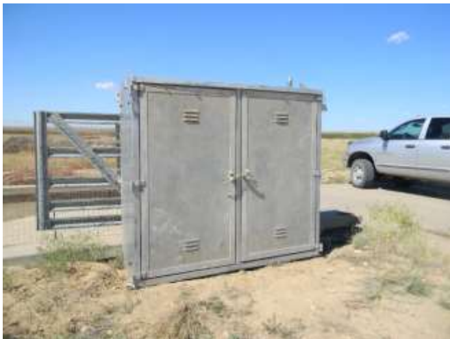
Figure 4 Railroad Signaling Cabinet repurposed as a storage locker
