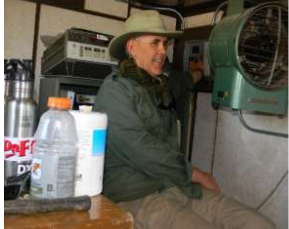
Figure 7 John Royo labeling the Comm Trailer circuit breakers
