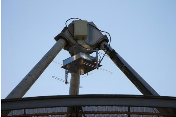
Figure 6: Multi-Band Feed Installed
